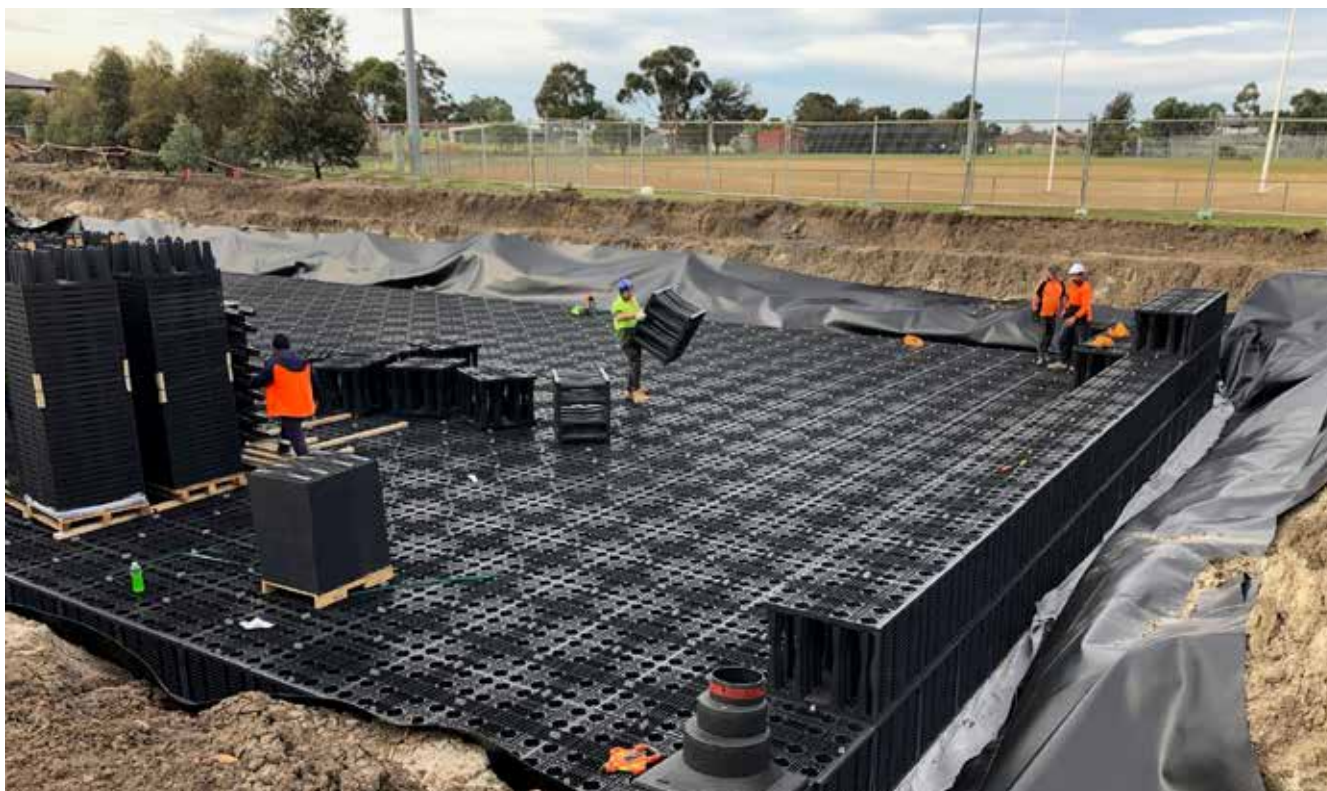
Stormwater Harvesting project at Dempster Park, Sunshine North
